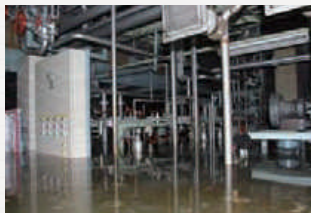
Inside the inundated plant at TJT (October 21, 2011)
